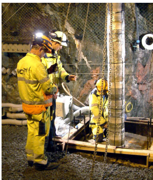
Installation of one of the three packages illustrating the mixing of the different compacted buffer discs.
